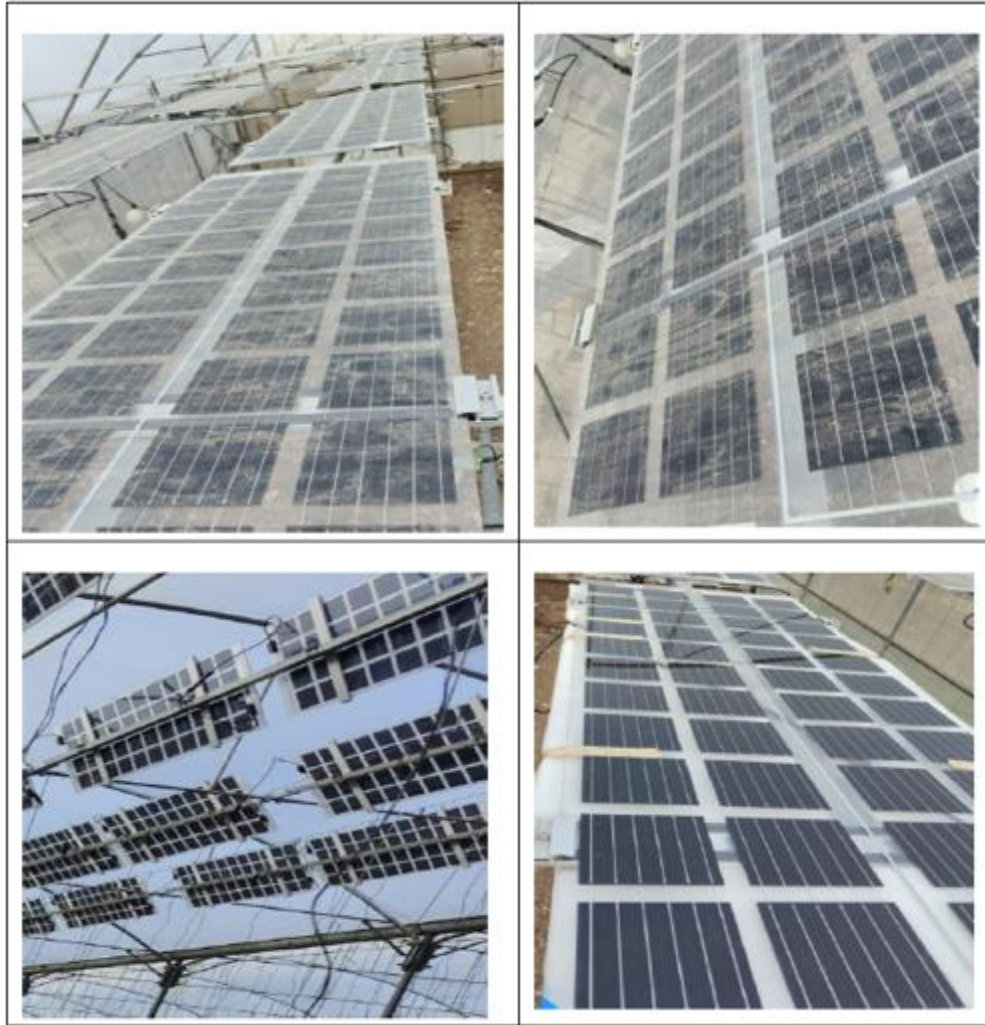
Figure 54. Dust accumulation on the PV cells.
