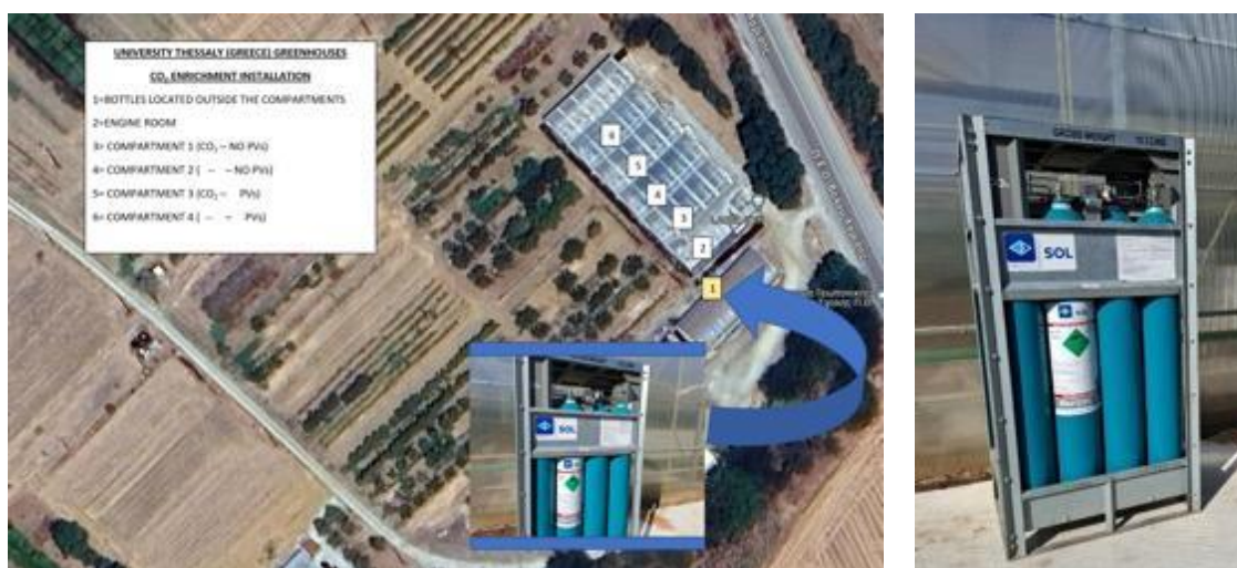
Figure 12 CO 2 cylinders placed outside the greenhouse
